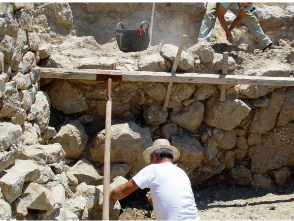
Figure 2. East wall of the Communal Dining Building, temporarily stabilized during conservation (Photo: Azoria Project)
