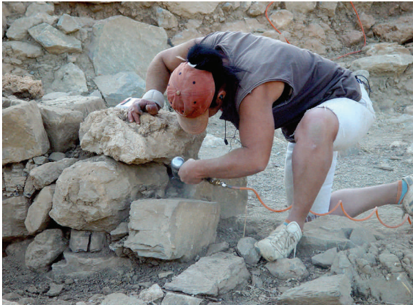
Figure 6. S. Papadaki using an air-compressor pistol to remove the ancient mortar. (Photo: Azoria Project)
