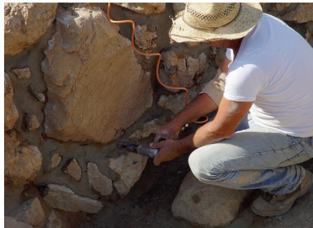
Figure 9. Use of the air-compressor pistol to pack the mortar (Photo: Azoria Project)
