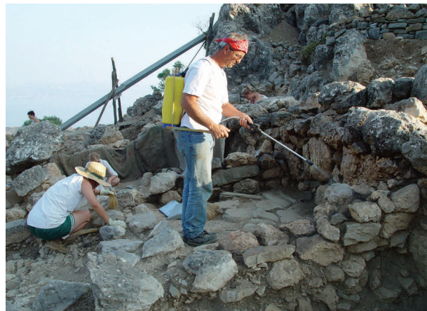
Figure 7. Excavation foreman M. Kasotakis washing a wall before application of the mortar (Photo: Azoria Project)
